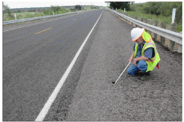
Note: Erosion hole approximately 3" in diameter and 4" from white stripe of Southbound lane and depth greater than 4" on SE end of bridge.
