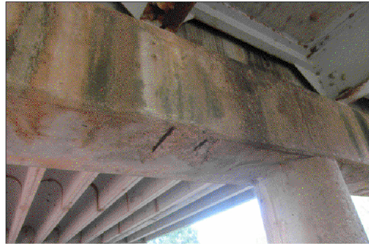
Note: Cap at bent 6 from NW has minor horizontal cracks along top edge and minor to moderate delaminations and spalls (up to 27"x18") with exposed rebar at underside.
