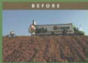
IH 20, Big Spring, Texas (loading slope erosion)
