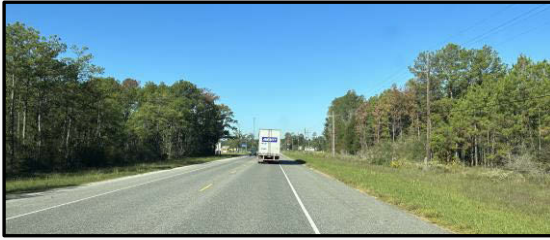
This photo shows the existing SH 105 roadway consisting of two 12-foot-wide travel lanes.
