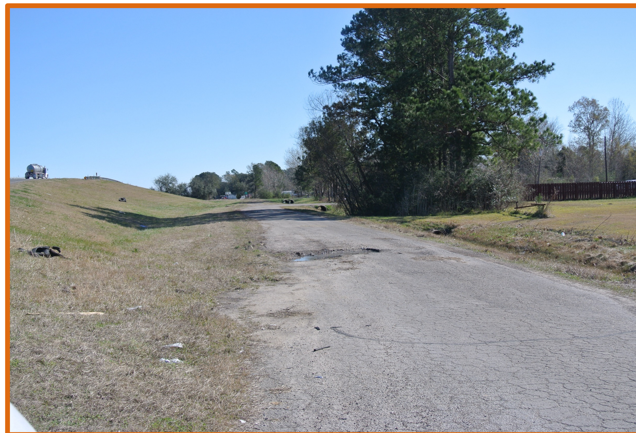
Existing frontage road condition
