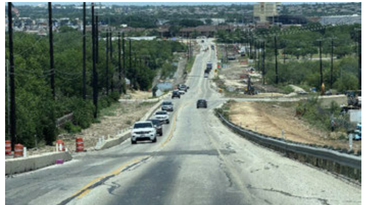
The two-lane roadway will soon become a five-lane roadway with a left-center turn lane and sidewalks.
