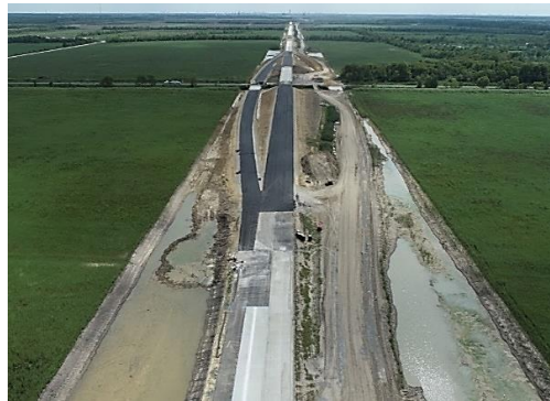
Figure A.5: HMA, Bond Breaker, and CRCP Placement at FM 1414 in Segment I1A
