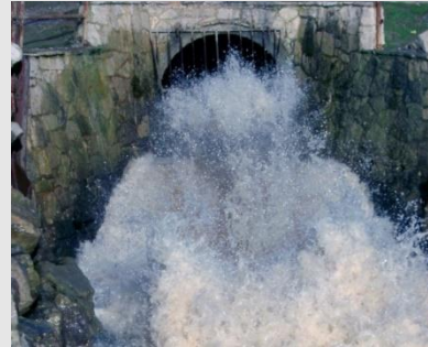
Culvert Failure; Overflows
