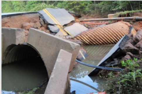
Culvert Failure; Structural Failure
