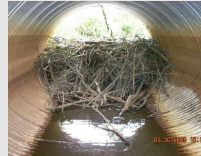
Culvert Failure; Blockages
